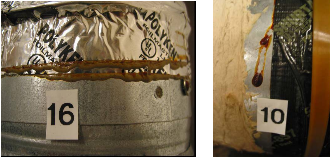
Figure 5. These samples show oozing of the adhesive at the tape edges.
